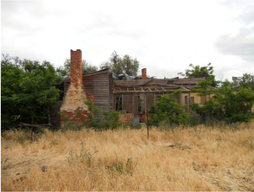
Plate 3.32: The eastern side of the building. The nearest chimney serviced a kitchen.
