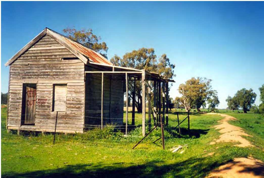
Plate 3.38: The former butcher shop and mission store photographed in 1993. (Heather Edwards collection)
