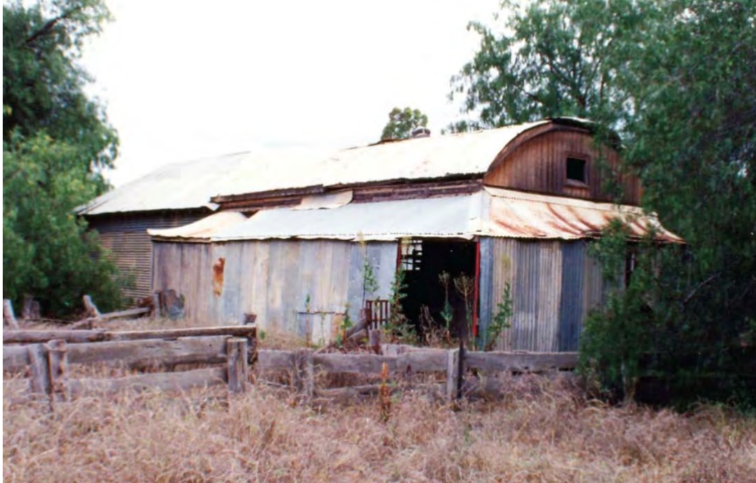
Plate 3.1: The Warangesda School building photographed from the northwest in 1993. A patch on the verandah roof indicates where the chimney was located. The large extension was a wool room for the woolshed. (Waddi Housing & Advancement Corporation)
