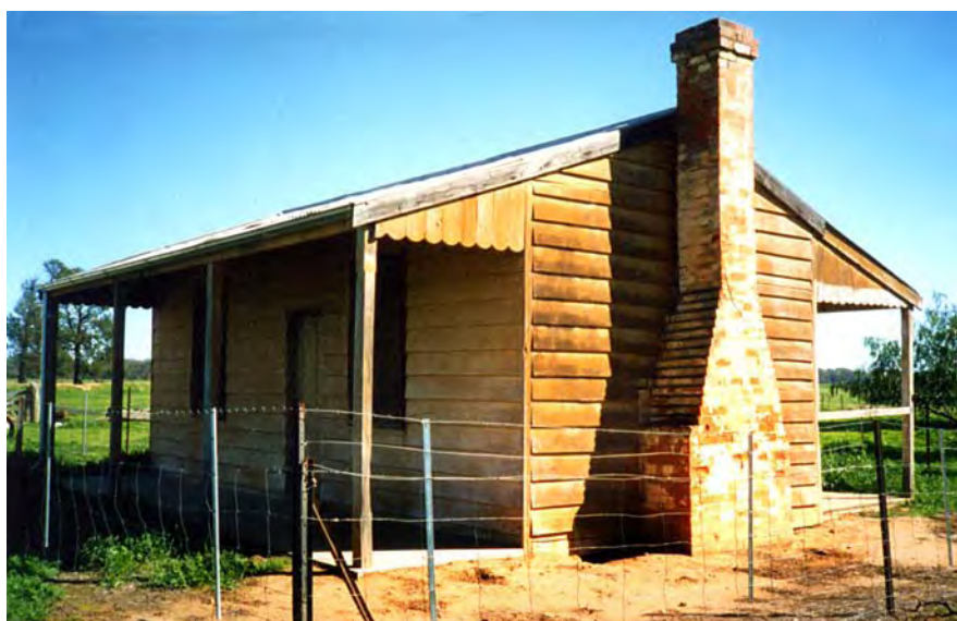
Plate 3.10: The 1898 teacher's house photographed in 2009 after conservation works. The bricks forming the chimney were subsequently stolen. (Heather Edwards collection)
