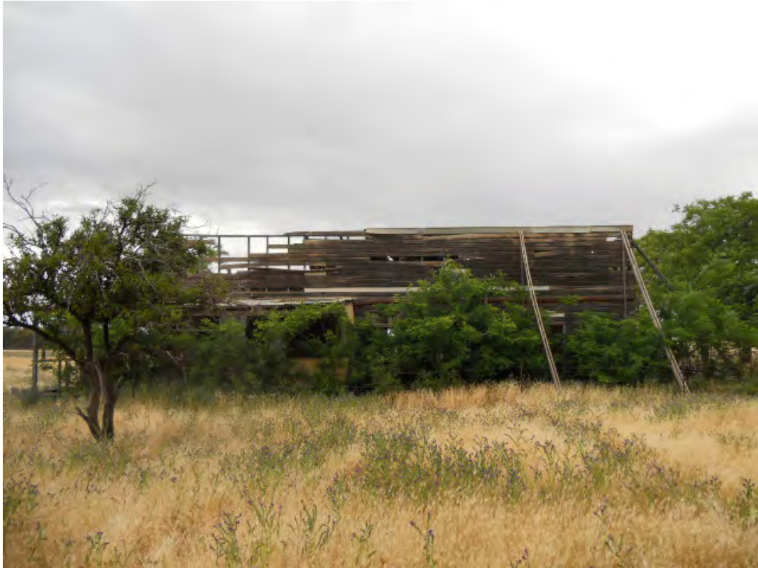
Plate 3.25: The western side of the former dormitory. This was the front of the building.
